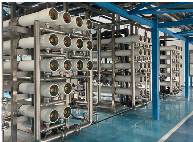
↑ Figure 2: Toray UF Unit (upper) and Toray RO Unit (lower)
